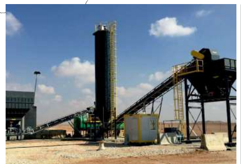
Cold / Wet Mix Plant
