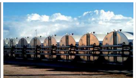
Tank, Piping and Insulation Systems
